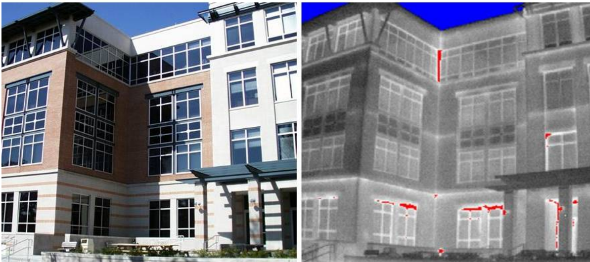
Figure 4. Visual and infrared image of an office building showing air leakage.
