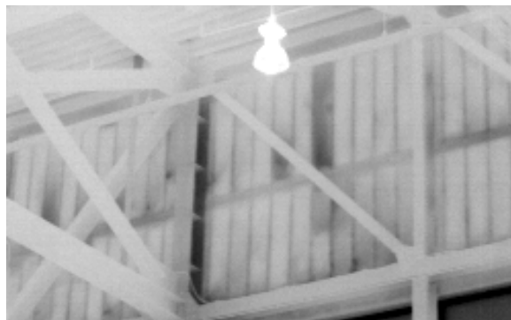
Figure 2. Infrared image of a convention center wall with missing and misplaced fiberglass batt insulation (darker areas).
