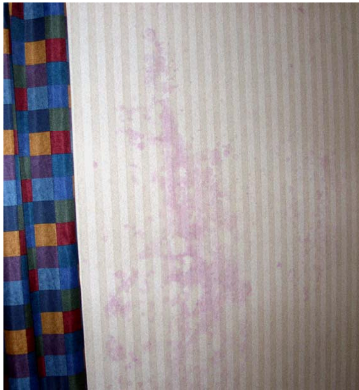
Figure 11. Visual image of the inside of a hotel outside wall with non-perforated vinyl wallpaper showing stains from mold.
