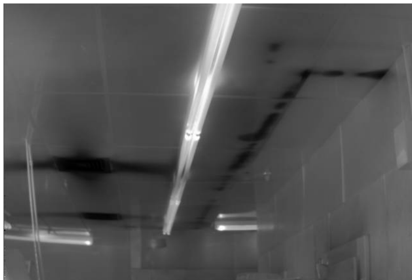
Figure 6. Infrared image of a restaurant kitchen, where uninsulated cold piping in the warm interstitial space drips water onto the ceiling.
